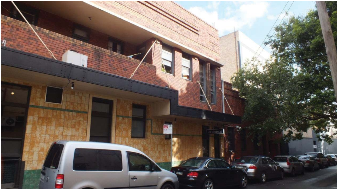
Figure 4 — the north-western elevation, sees from Dunblane Street. Cracks in the brickwork may indicate deflection in the concrete slab. NBRSPARTNERS April 2014
