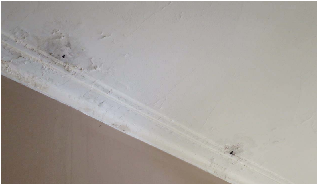
Figure 11 — view of water damage to ceiling at the western end of the first floor hall.
