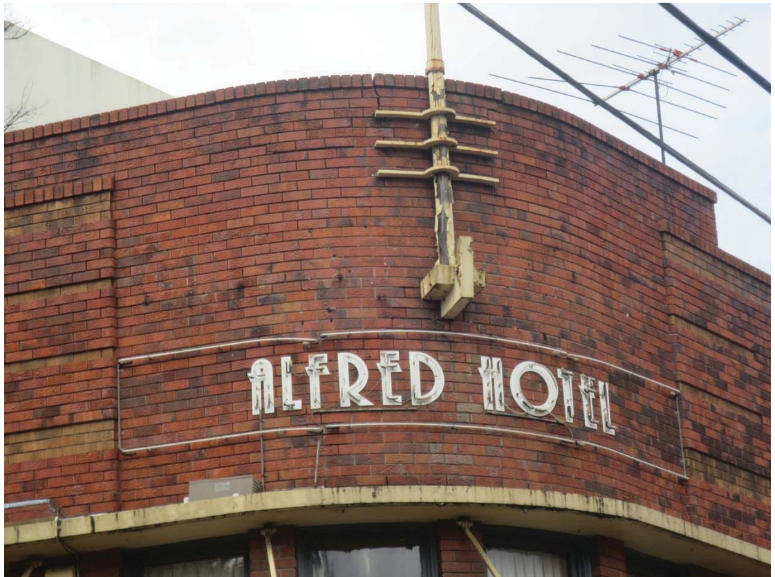
Figure 6 — cracks in the parapet are likely caused by rusting steel fixings attaching the flagpole.
