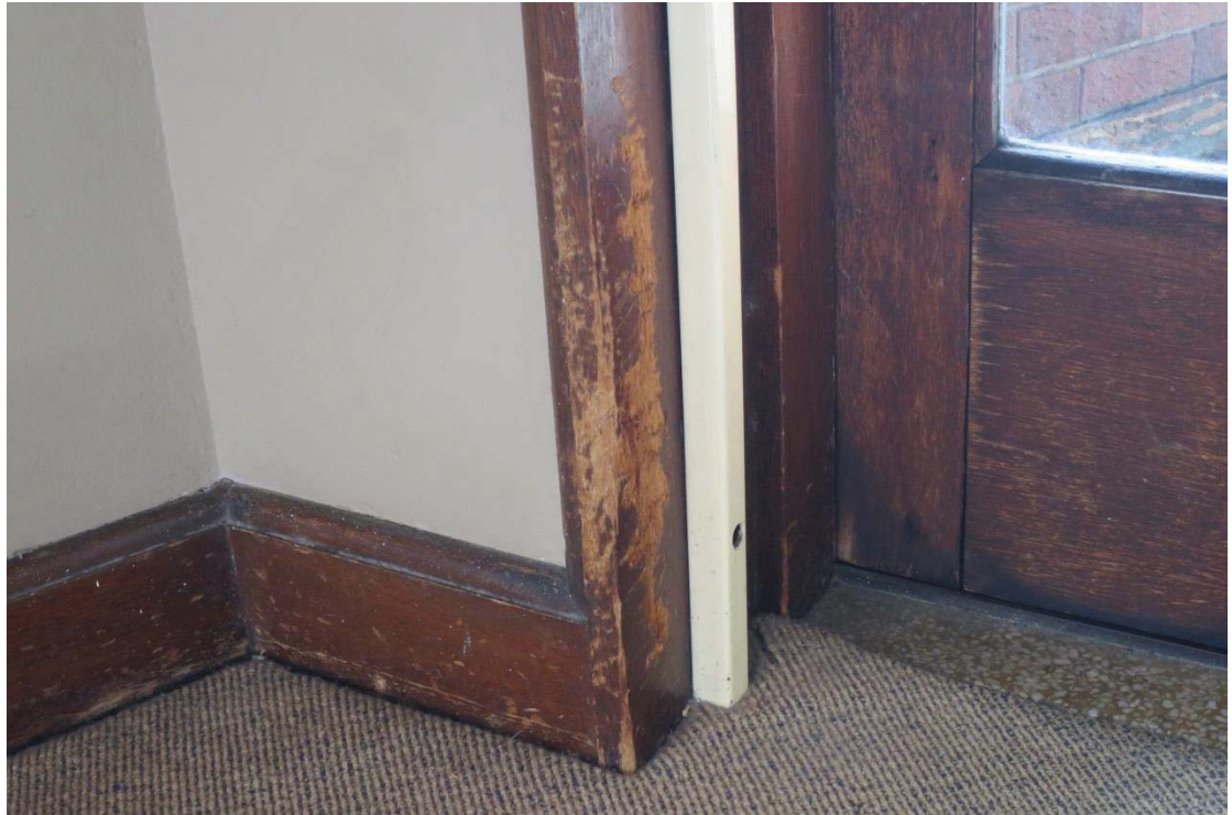
Figure 12 — impact damage to a simple section of meranti joinery in the first floor bedroom with a curved corner. Joinery elements with this degree of damage should be replaced to match.
